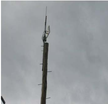
Figure 6. AP and panel antenna at Mugumu Distribution Point
