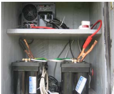
Figure 8. Backup power system
